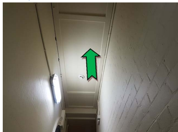
Photo 6. Interior, level one, north stairs, ceiling – suspected asbestos-containing fibre cement sheeting.
