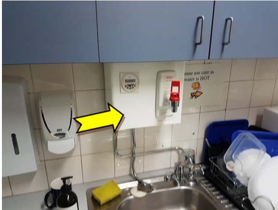
Photo 13. Interior, ground level, north-west elevation, kitchen, hot water heater – suspected SMF internal insulation material.
