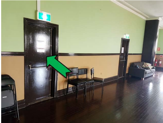
Photo 1. Interior, throughout, fire doors – suspected non asbestos-containing fire door core.
