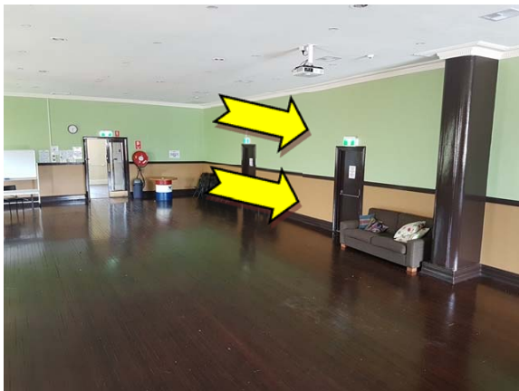
Photo 15. Interior, level one, hall, walls – suspected lead-containing green, beige and brown upper coloured paint systems.
