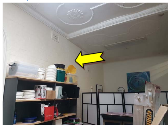
Photo 18. Interior, throughout, walls – suspected lead-containing white upper paint systems.
