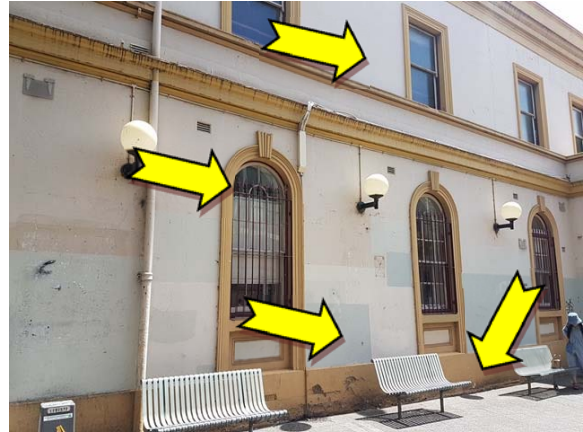
Photo 14. Exterior, throughout, walls and window frames – suspected lead-containing beige, yellow, red and white upper coloured paint systems.
