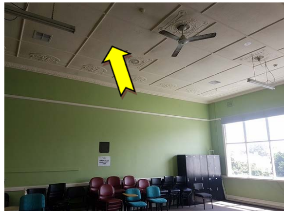
Photo 16. Interior, level one, throughout, ceiling – suspected lead-containing white upper paint systems.
