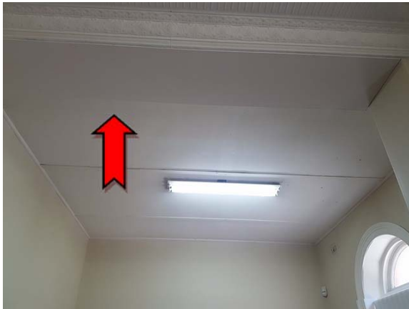
Photo 9. Interior, ground level, reception office, ceiling – suspected asbestos-containing fibre cement sheeting.
