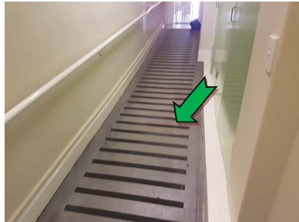
Photo 10. Interior, ground level, central ramp, grey floor coverings – non asbestos-containing vinyl sheeting.
