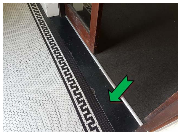
Photo 12. Interior, ground level, entrance, black floor coverings – non asbestos-containing vinyl floor tiles.
