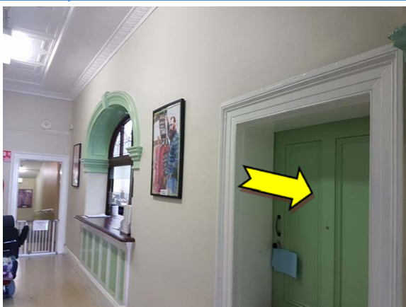
Photo 17. Interior, throughout, door – suspected lead-containing green upper paint system.
