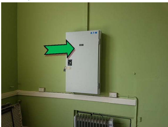
Photo 5. Interior, level one, electrical backing board – suspected non asbestos-containing bituminous backing board.
